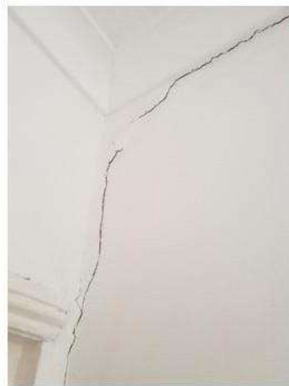
Image 01- Wall cracks due to ground instability
